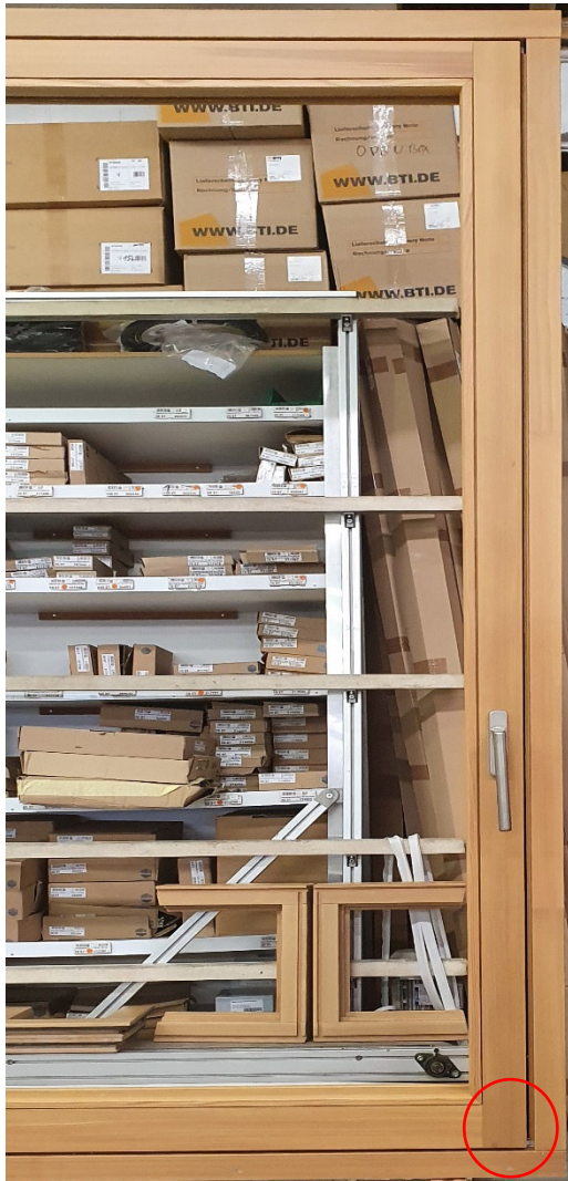
Gap wider at bottom
